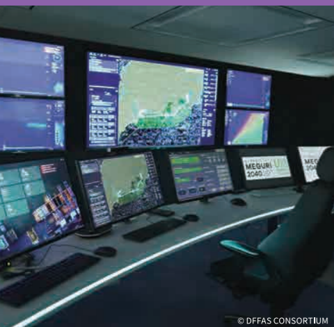
Fleet Support System Console
